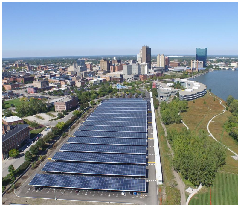
The solar carport at the Owens Corning headquarters in Toledo, OH has a total installed capacity of 2.4 MW; Photo: Owens Corning
