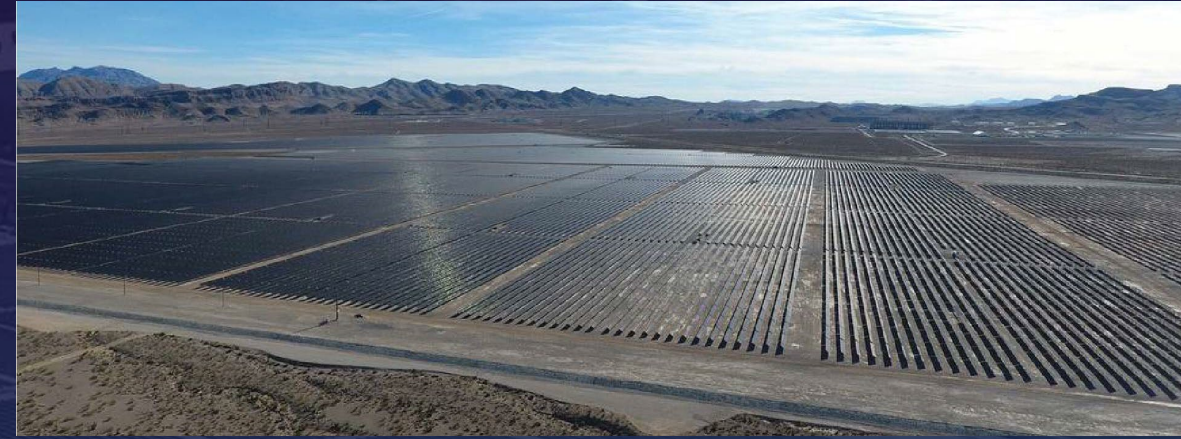
Photo Courtesy of Switch
