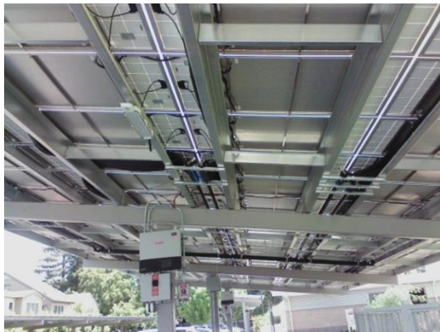
Collectors visible underneath the carport.
