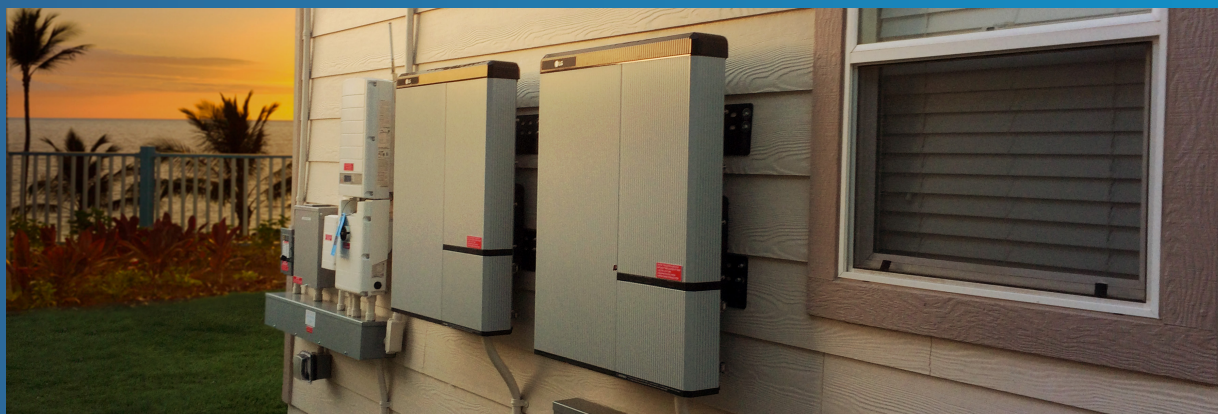
Home energy storage systems help support a resilient, reliable and sustainable electric grid. Photo courtesy of Sunrun, Inc.
