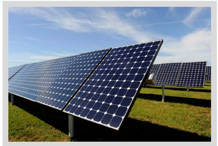
The 25 MW photovoltaic DeSoto Next Generation Solar Energy Center in DeSoto County, Fla., was completed in October 2009.
